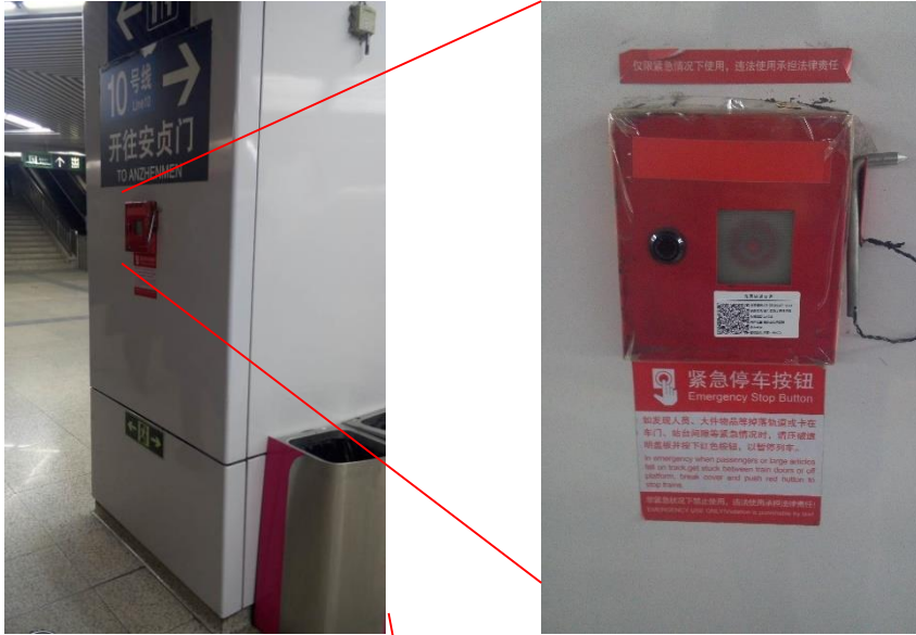
Emergency button on platform
