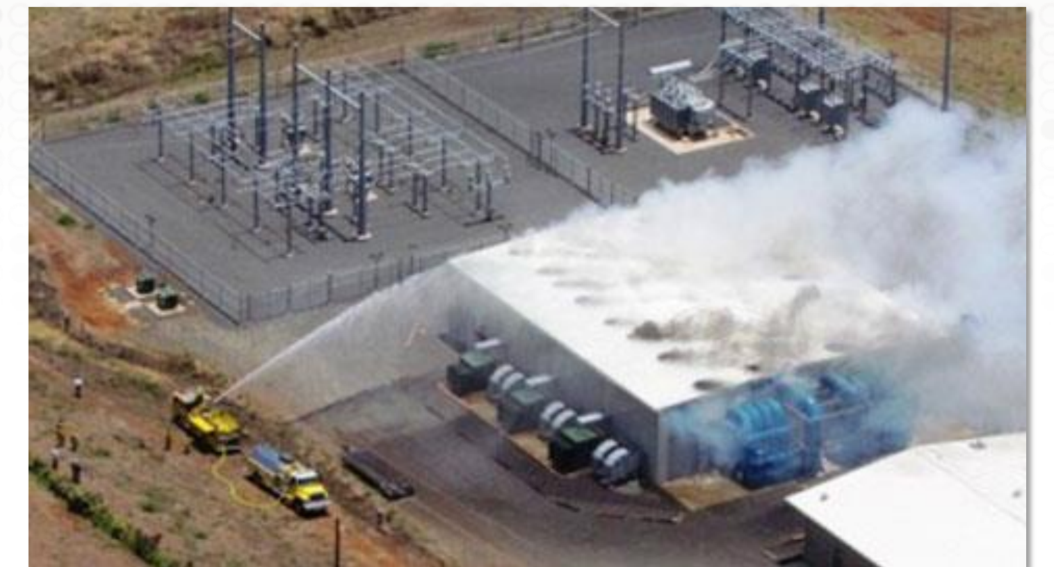
Figure 1 Battery Fire at Kahuku Wind-Energy Storage Farm, Oahu Hawaii, August 1st 2012 (From www.hawaiinewsnow.com courtesy: Jay Armstrong)
