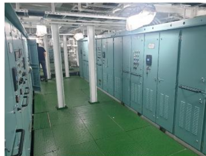
Power distribution panels
