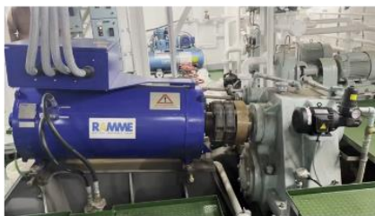
Propulsion motor test w/ battery
